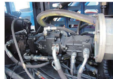
泵组 Pump group
